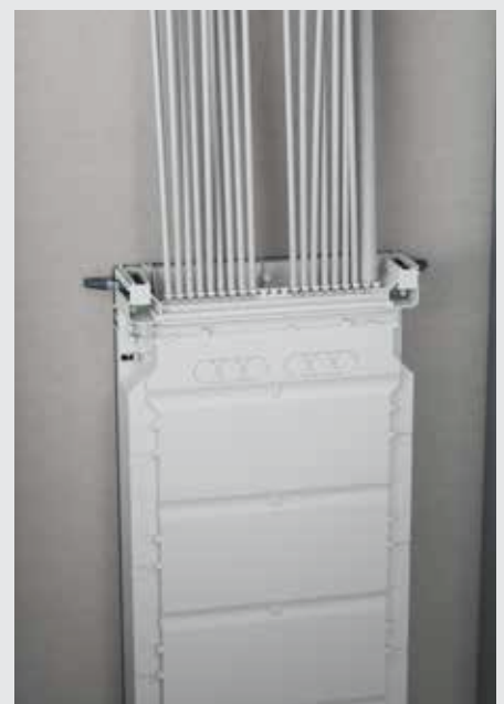
The central transition casing for the exit of several cables.
